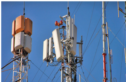
Figure 3. Base transceiver station (BTS)
