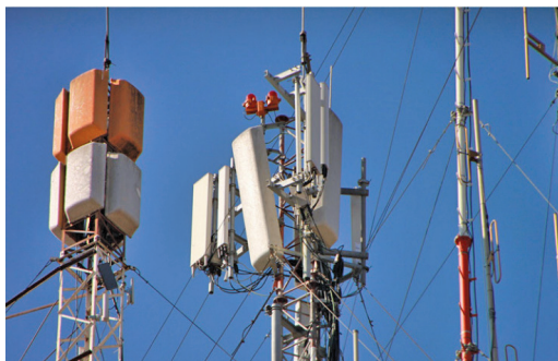
Figure 3. Base transceiver station (BTS)
